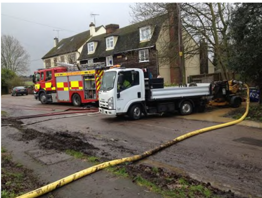
Figure 2: Emergency pumping of flood water
